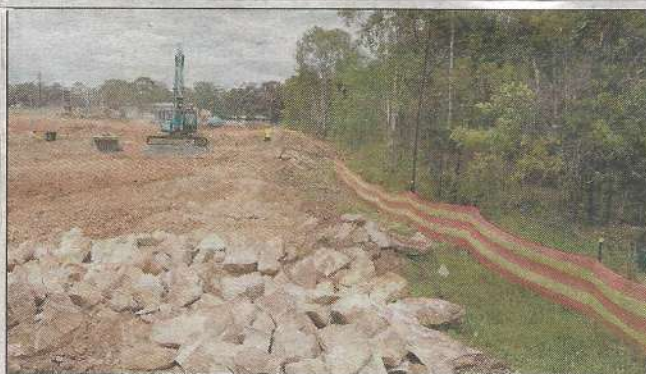
Bulldozers continue land clearing along Smiths Creek Reserve bush corridor in Airds last week.
